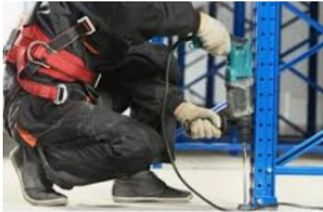
The hole for the anchor bolt is drilled through the baseplate of the assembled, spotted, and leveled rack.
